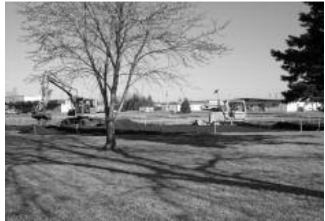
Village street employees construct the new Farmers’ Market Park scheduled to open June 4 th . (Photo: Tim Vergara)
